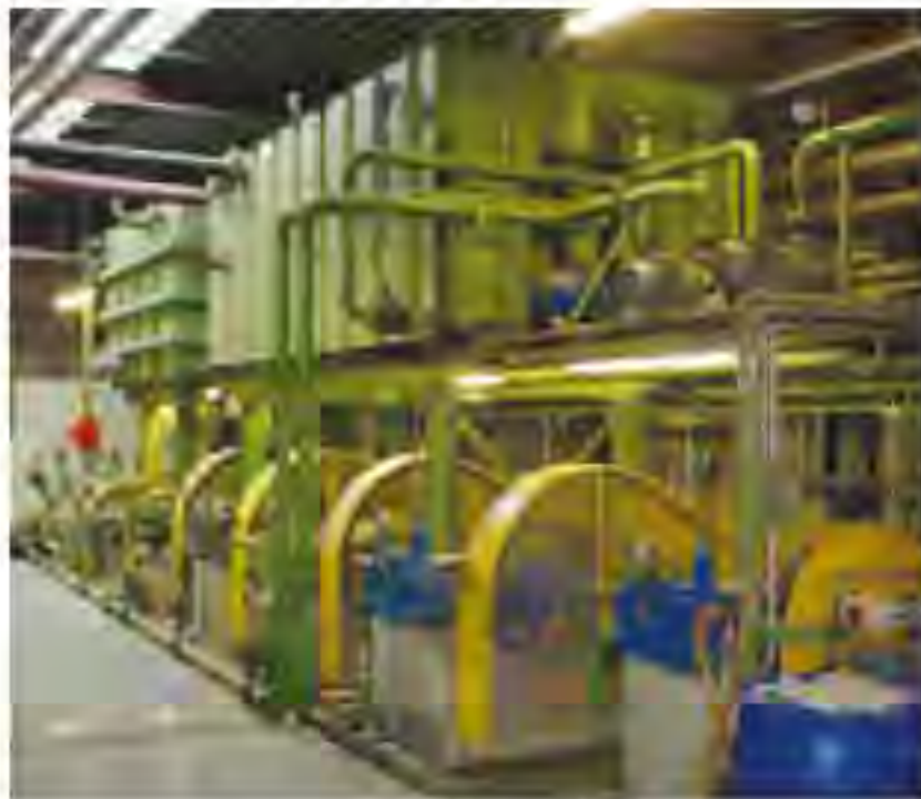
Pump units in a pressurized water system.
