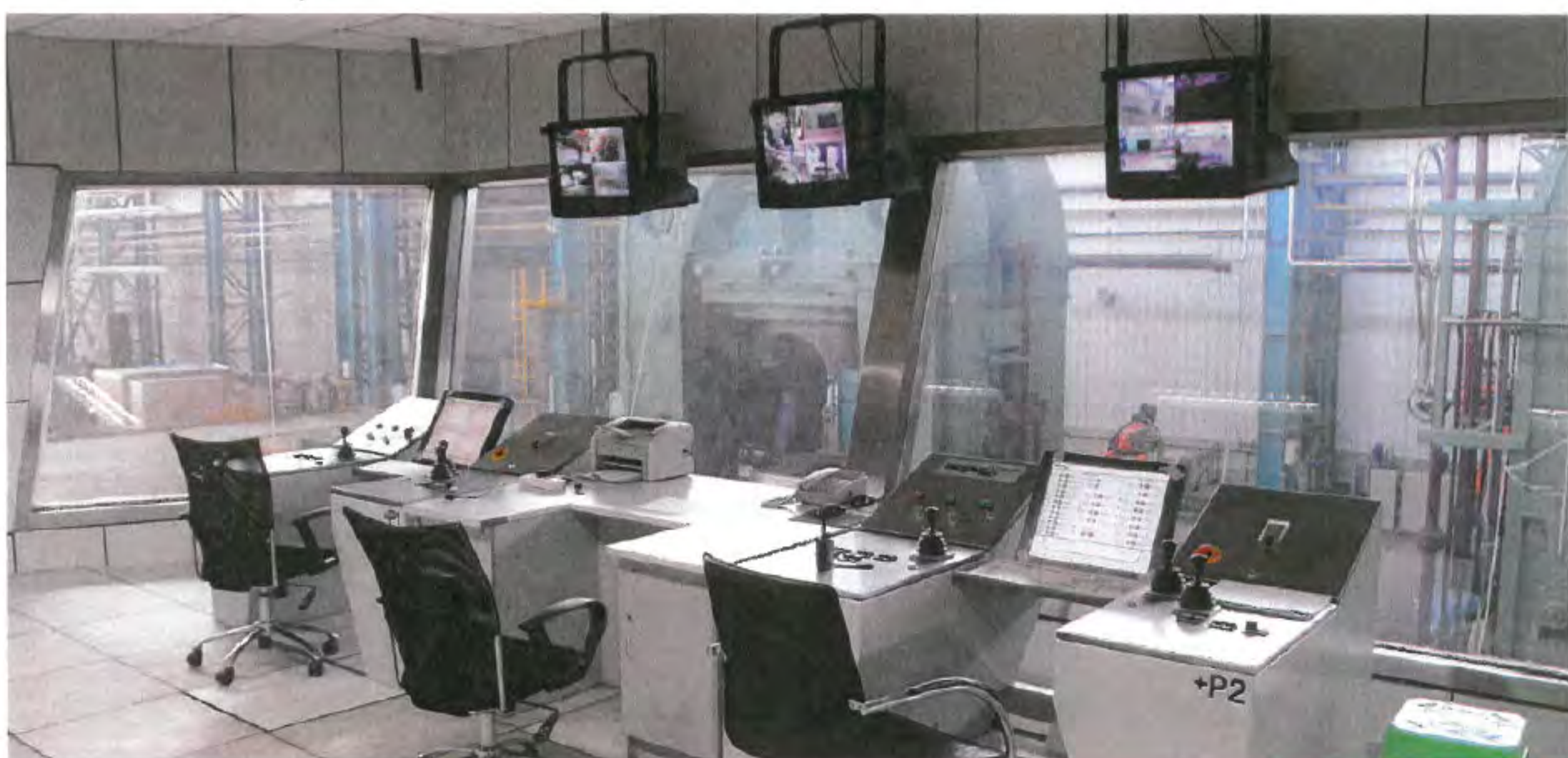
Control room for a 360 MN steel extrusion press and a 150 MN preforming press.
