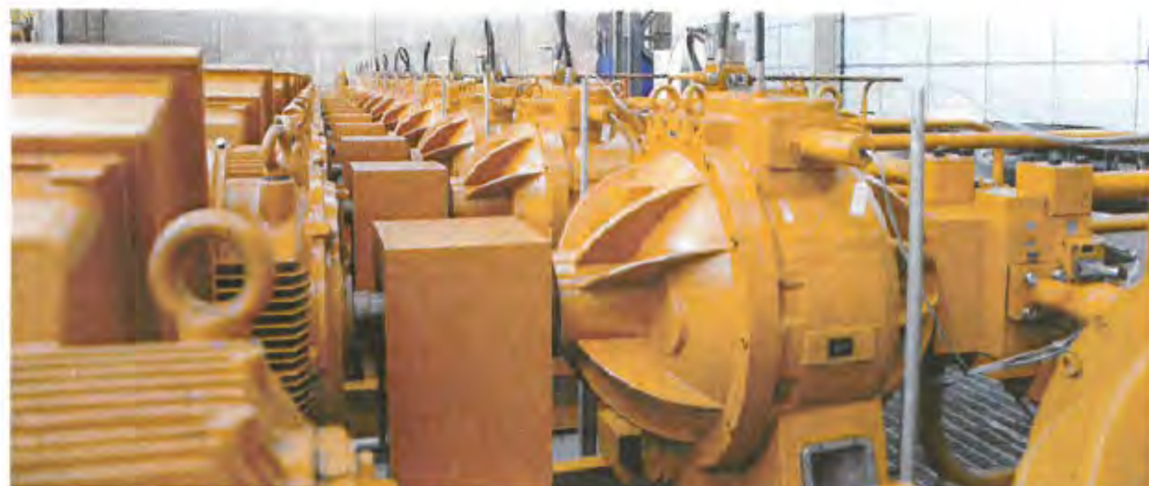
16-pump PMSD drive (RX 500) of an 80/100 MN press.
