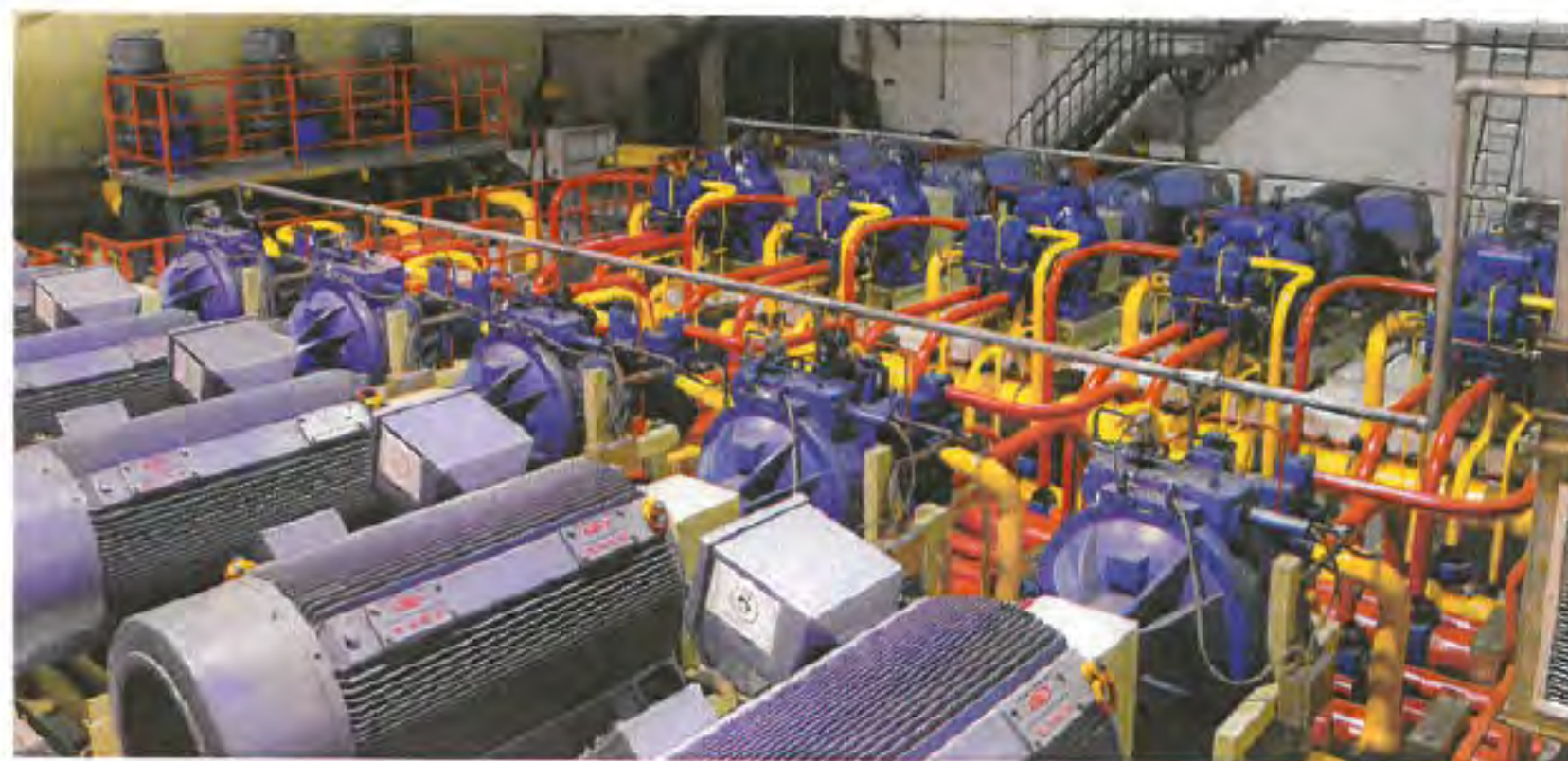
Part of the 20-pump PMSD drive (RX 500) of a 185 MN press.
